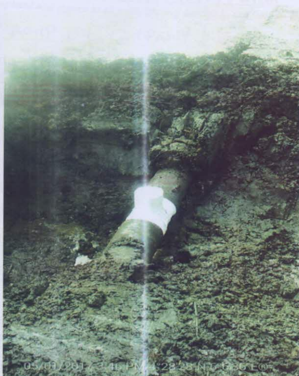
INTERFERENCE POINT AFTER REPAIR
